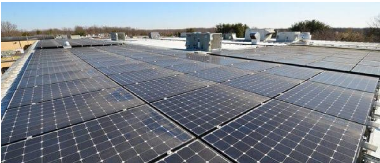
Figure 28: Solar Panels atop Interstate Packaging, Hwy 47N, White Bluff, TN
